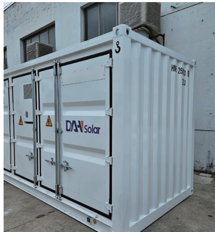
Installed capacity: 110MWh Product specification: 5MW / 10MWh Containerized Energy Storage System
