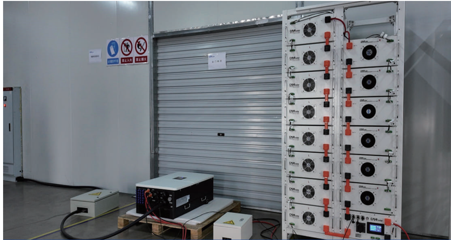
Installed capacity: 200kWh Product specification: 80kW / 200kWh High Voltage Energy Storage System
