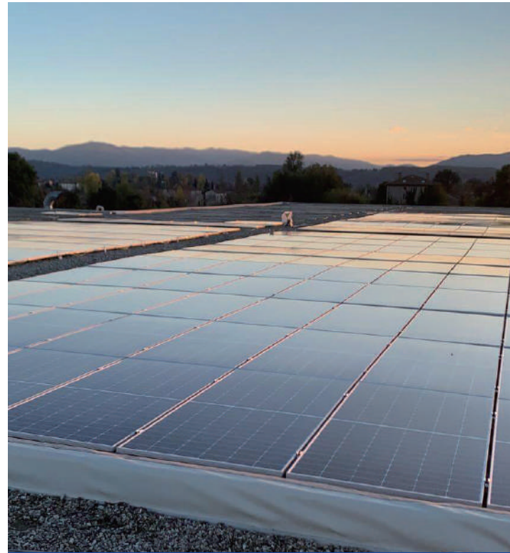
Installed capacity: 200kWh Product specification: Hybrid Inverter + Lithium Battery
