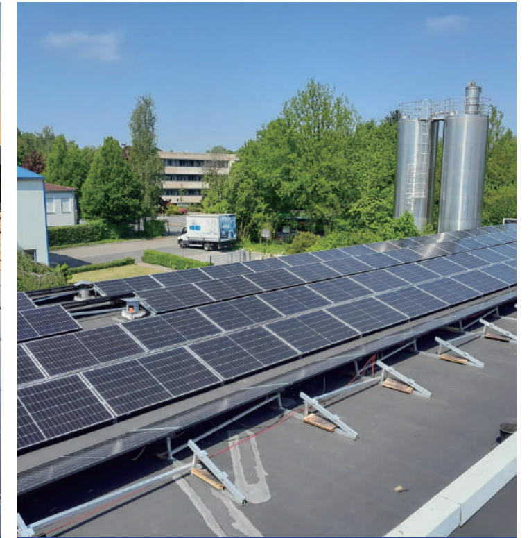
Installed capacity: 100kWh
